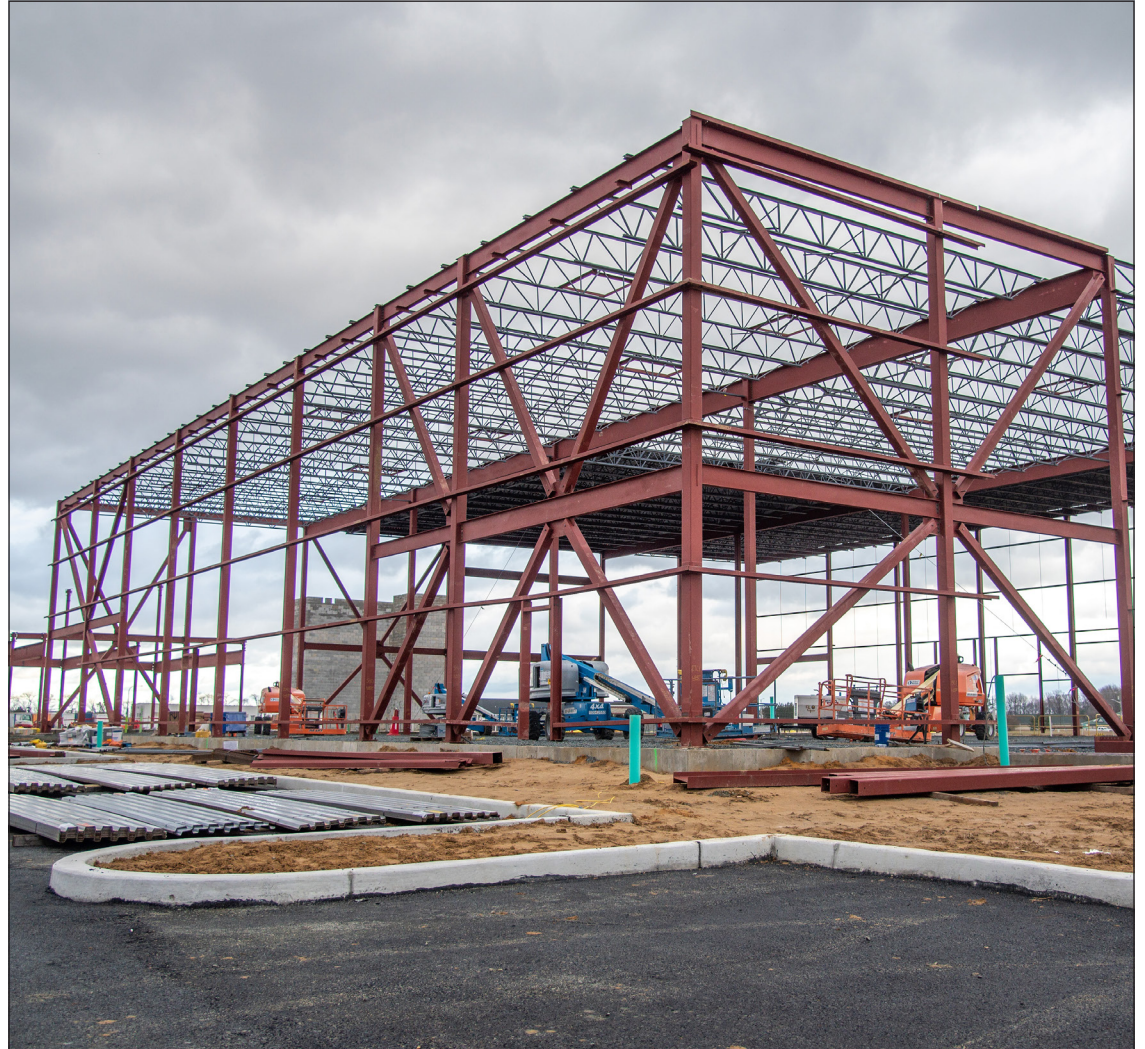
Steel framework at the construction site of the Food Bank of Delaware facility in Milford on Monday.
