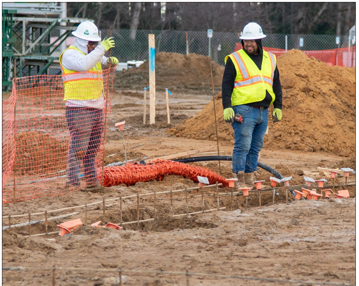
Workers at the Food Bank of Delaware construction site in Milford on Monday. DELAWARE STATE NEWS/MATT MCDONALD
